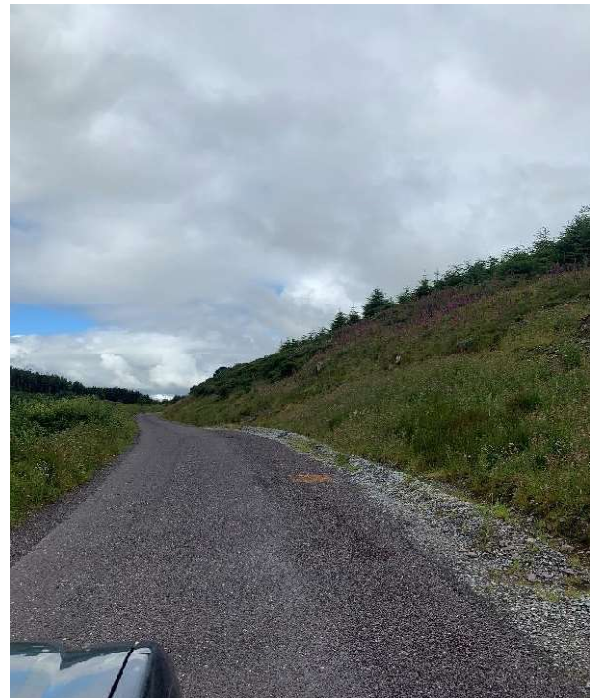
Image : 16 Joint bay on the road here with a links box and communications chambers visible.
