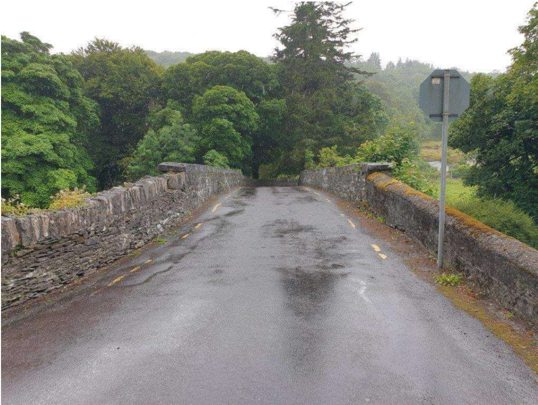
Road surface showing wear, abrasion and some rutting
