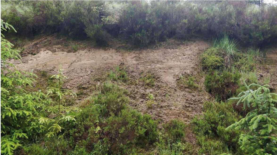
Figure 6-6: Exposed overburden cut with evidence of erosion/shallow slips (ITM 516203E,582880N)
