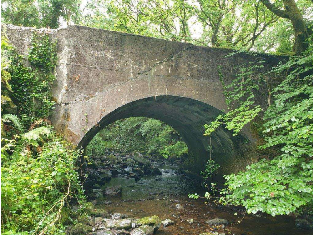
General view of the south elevation, note damage to parapet and west spandrel
