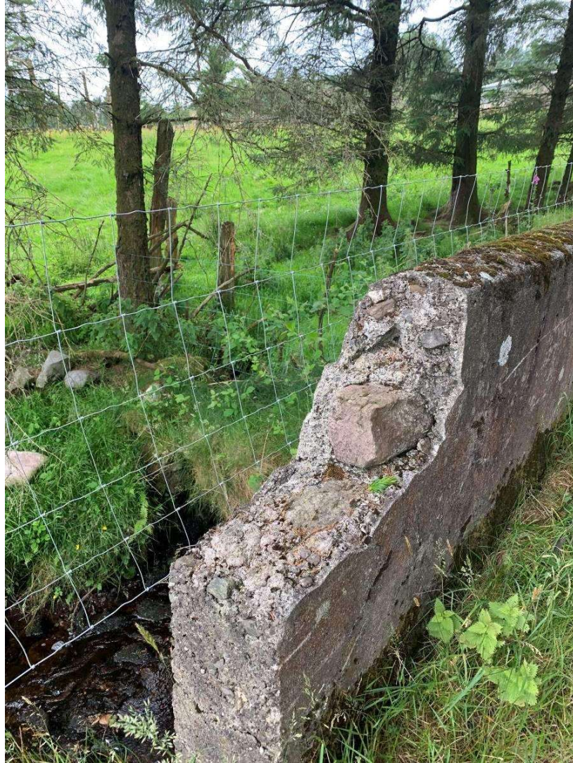
Knocked section of the downstream parapet
