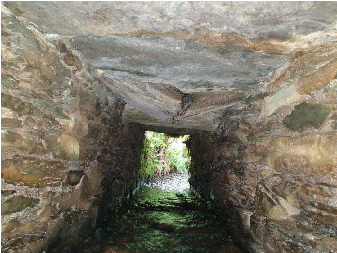
Soffit of bridge deck/box stone culvert. Flag stone is damaged and has collapsed as seen viewed from U/S (north span).
