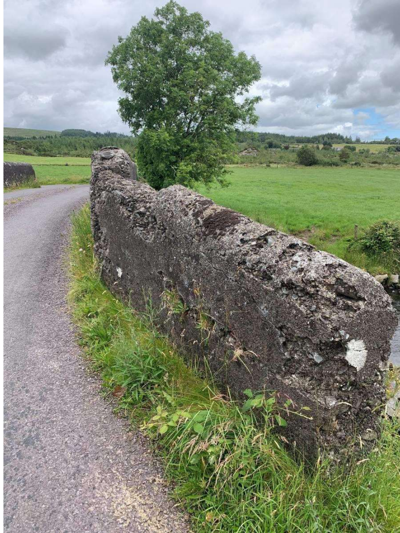
Close up of parapet showing concrete damage
