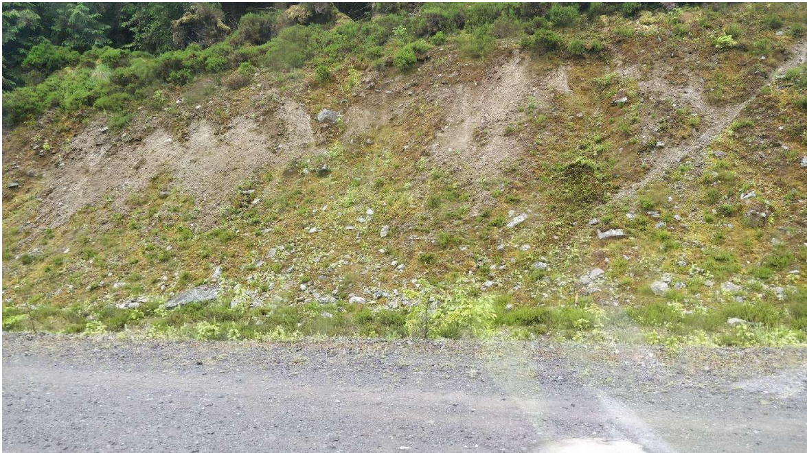
Figure 6-7: Exposed overburden cut with evidence of erosion/shallow slips (ITM 519555E,583500N)
