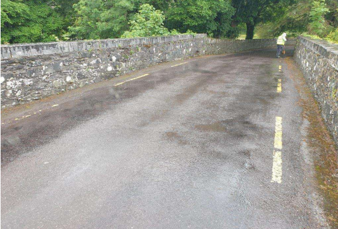
Road surface showing wear, abrasion and some rutting
