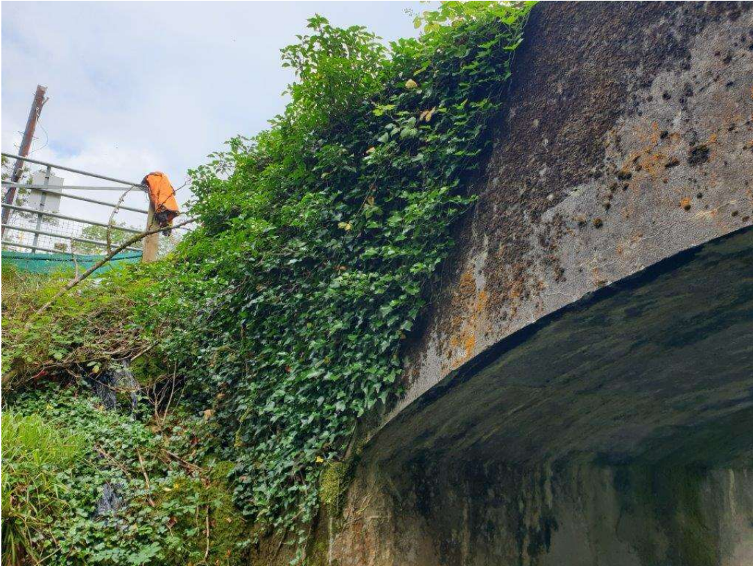
Vegetation growth on the west elevation
