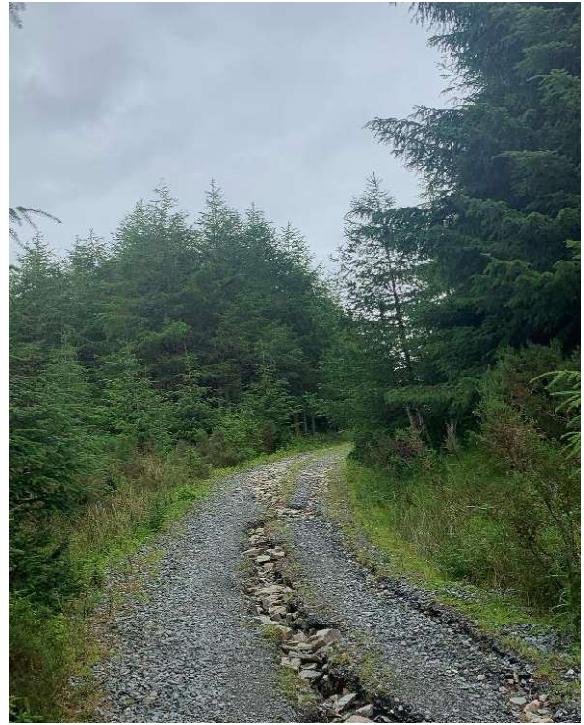
Image : 73 Forestry track on Coillte lands very step and heavily rutted
