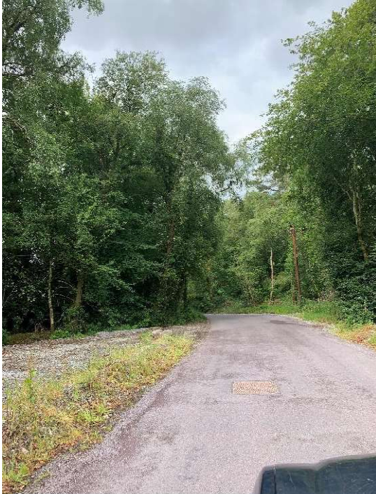
Image : 37 Joint bay on the road here with a links box and communications chambers visible.
