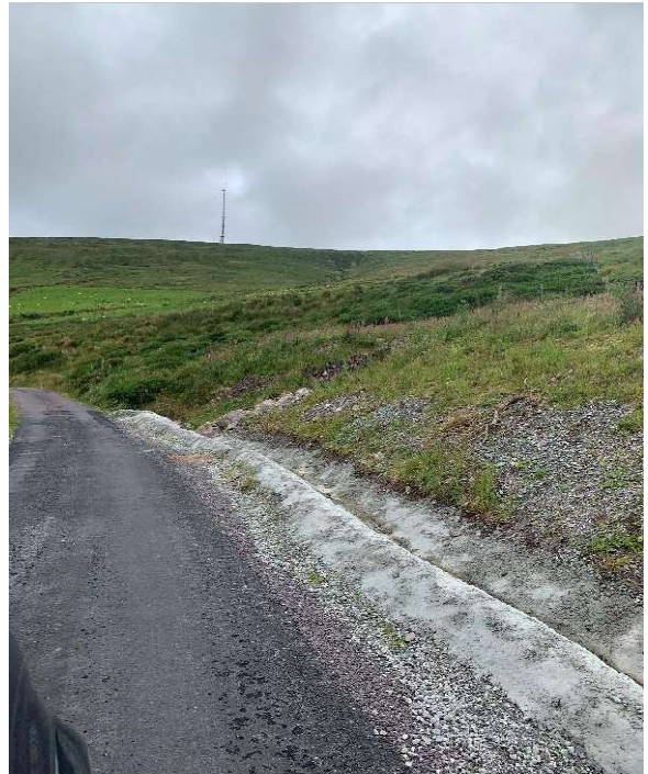
Image : 18 Joint bay on the road here with a links box and communications chambers visible.
