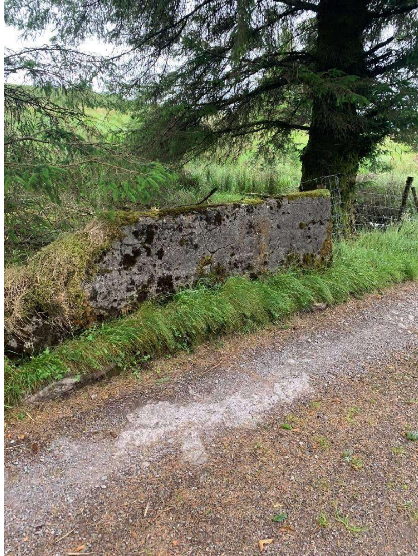
Upstream parapet with knocked section and structural cracking
