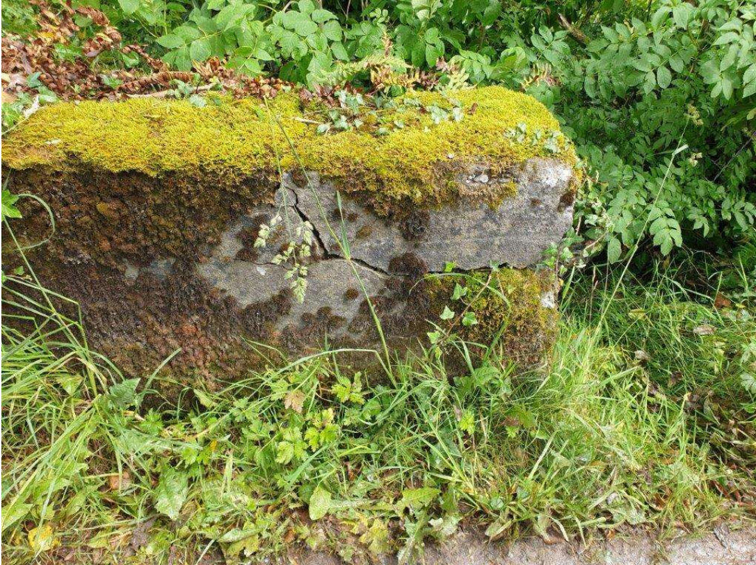
Local damage to the west parapet
