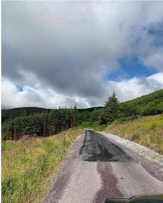
Image : 13 Possible location of joint bay which has had the covers tarred over.
