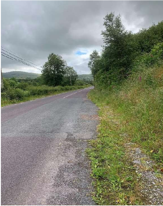
Image : 41 Joint bay on the road here with a links box and communications chambers visible.
